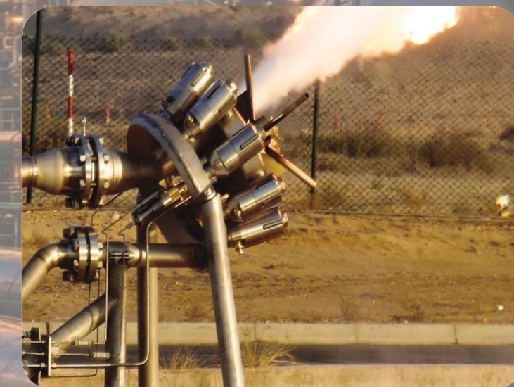
Burner Heads & Ignition System
