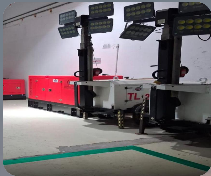
Electric Generators & Tower Lights
